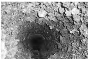
A pipeline prior to line pigging.
