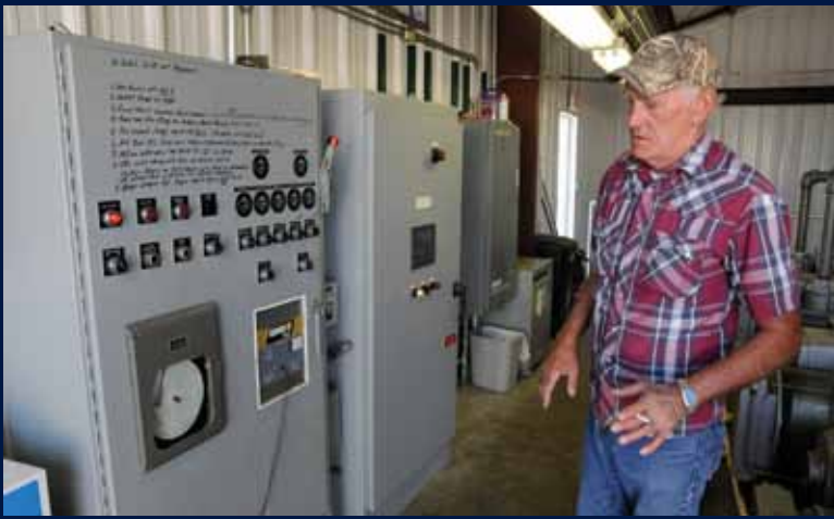
Plant supervisor Don Jones checks the wastewater operations control panel.
